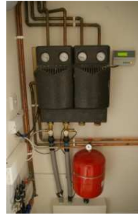
Figure 3.14 Ground floor under stairs controls
