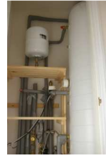
Figure 3.15 Upstairs hot water
